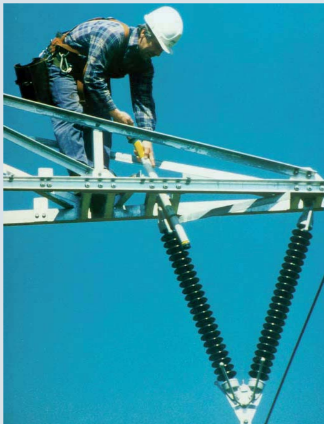
Non-contact voltage detector used for a 110 kV overhead line
