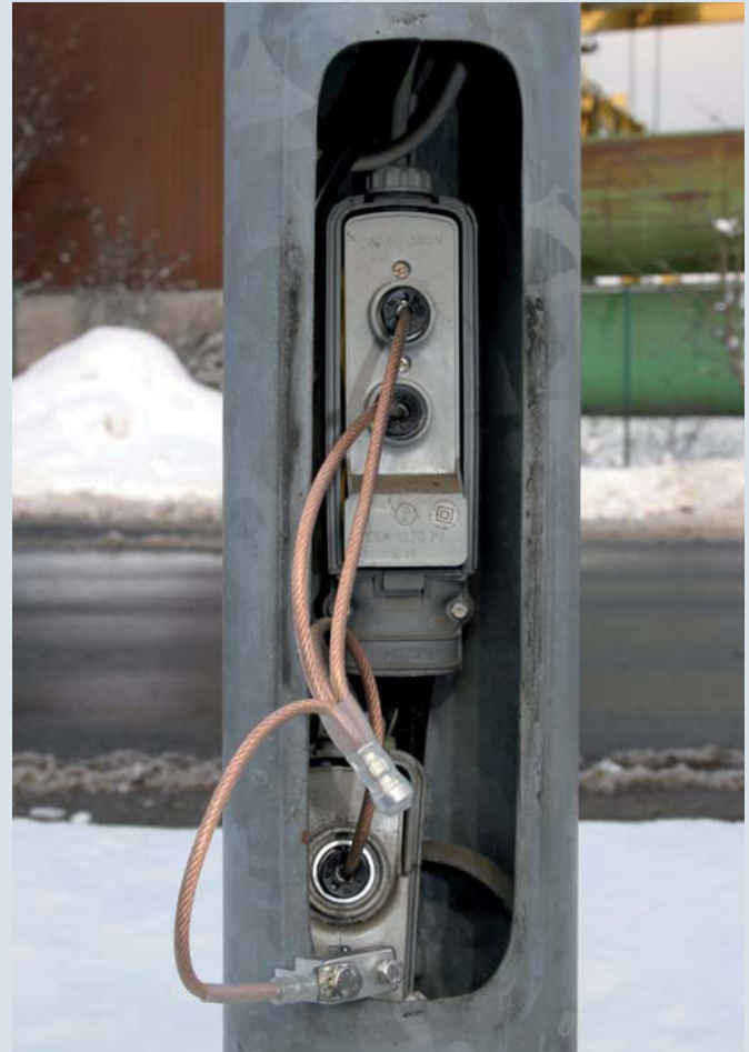
Earthing and short-circuiting device installed at a junction and fuse box of a street lighting mast
