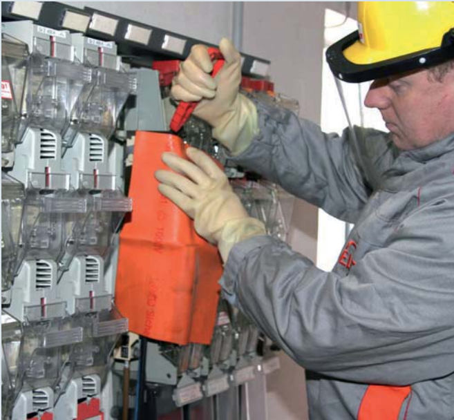
Live working with insulating gloves up to 1000 V
