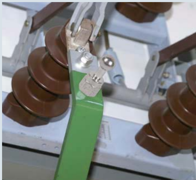
Straight fixed ball point mounted on a busbar
