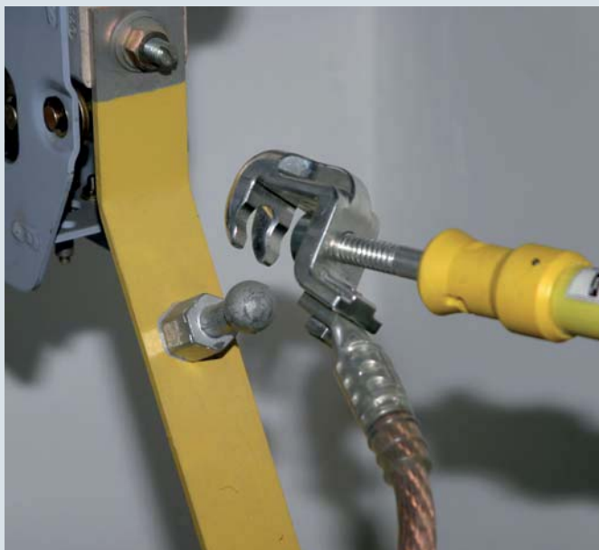
Connecting the phase cable end with universal clamp to a fixed ball point
