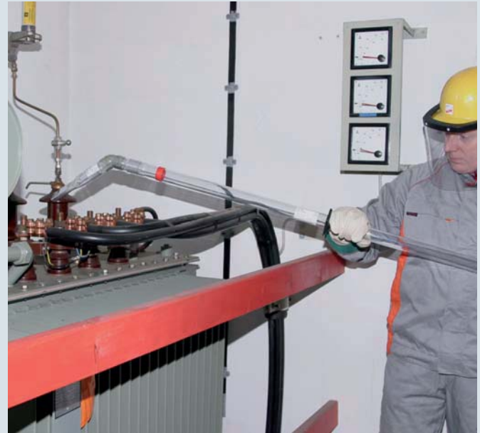
Live cleaning of a transformer using the TRS MS dry cleaning kit
