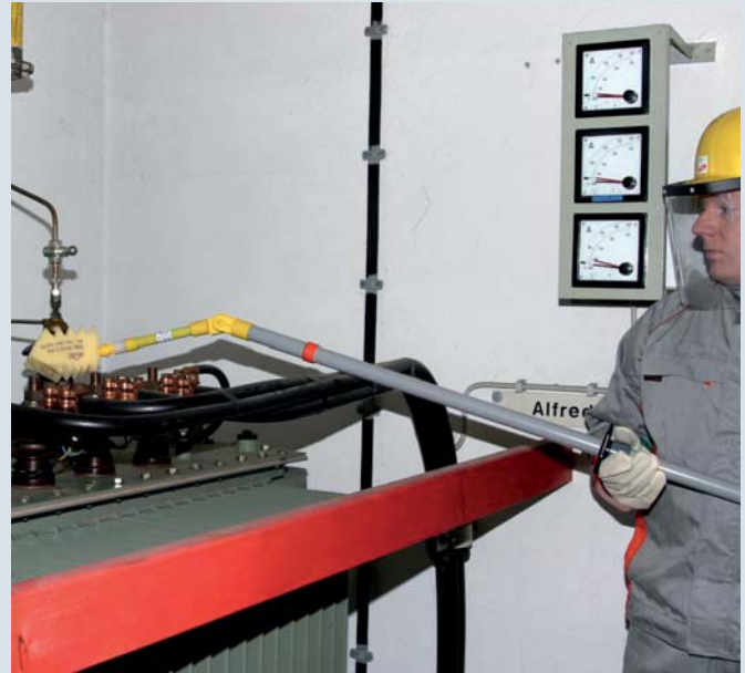
Damp cleaning of a transformer using the FRS ZK MS damp cleaning kit
