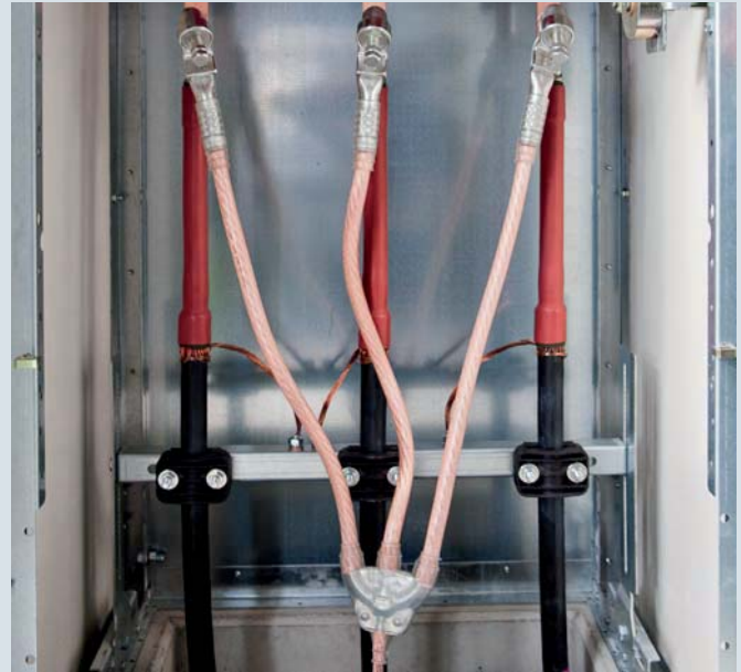
Equipped three-pole earthing and short-circuiting device in a switchgear installation
