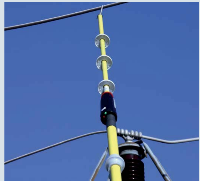
PHE III voltage detector used on a 110 kV outdoor switching station
