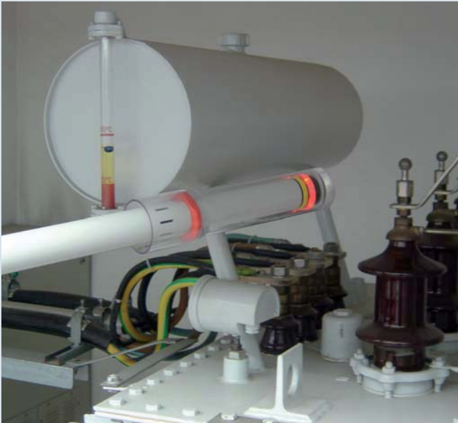
HSA 205 non-contact voltage detector with insulating cap used on a switchgear installation
