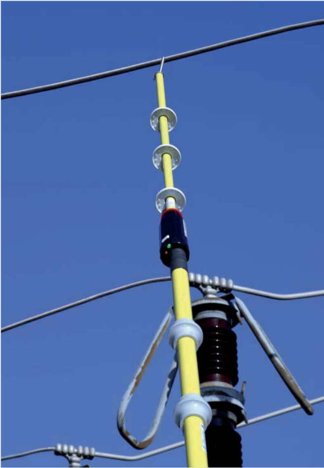
PHE III voltage detector used on a 110 kV outdoor station
