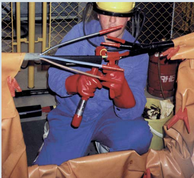
Covering live parts
