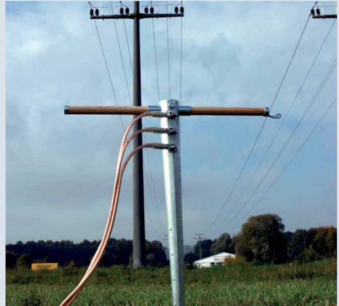
Earthing busbar and earthing cables mounted on a tubular earth electrode
