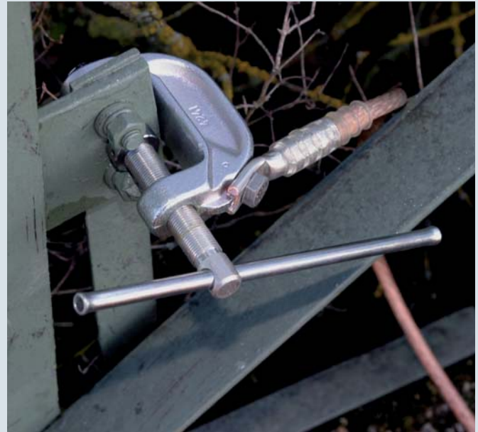
Earth milling clamp used on a coated steel tower
