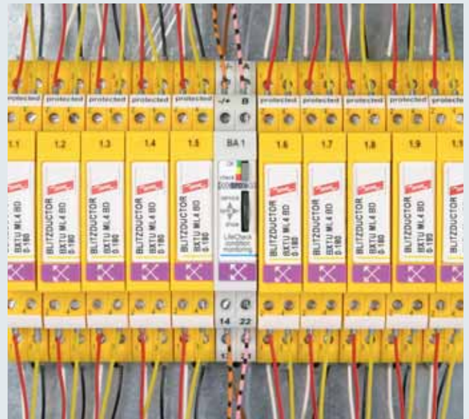
Installed DEHNrecord condition monitoring unit
