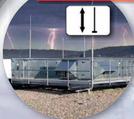
DEH Air-Termination Tool - Page 19 Calculation of the length of the air-termination rods in accordance with EN 62305-3
