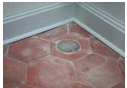
Top: cassette solution in an old building Above: GESRM2 in historical tiled floor
